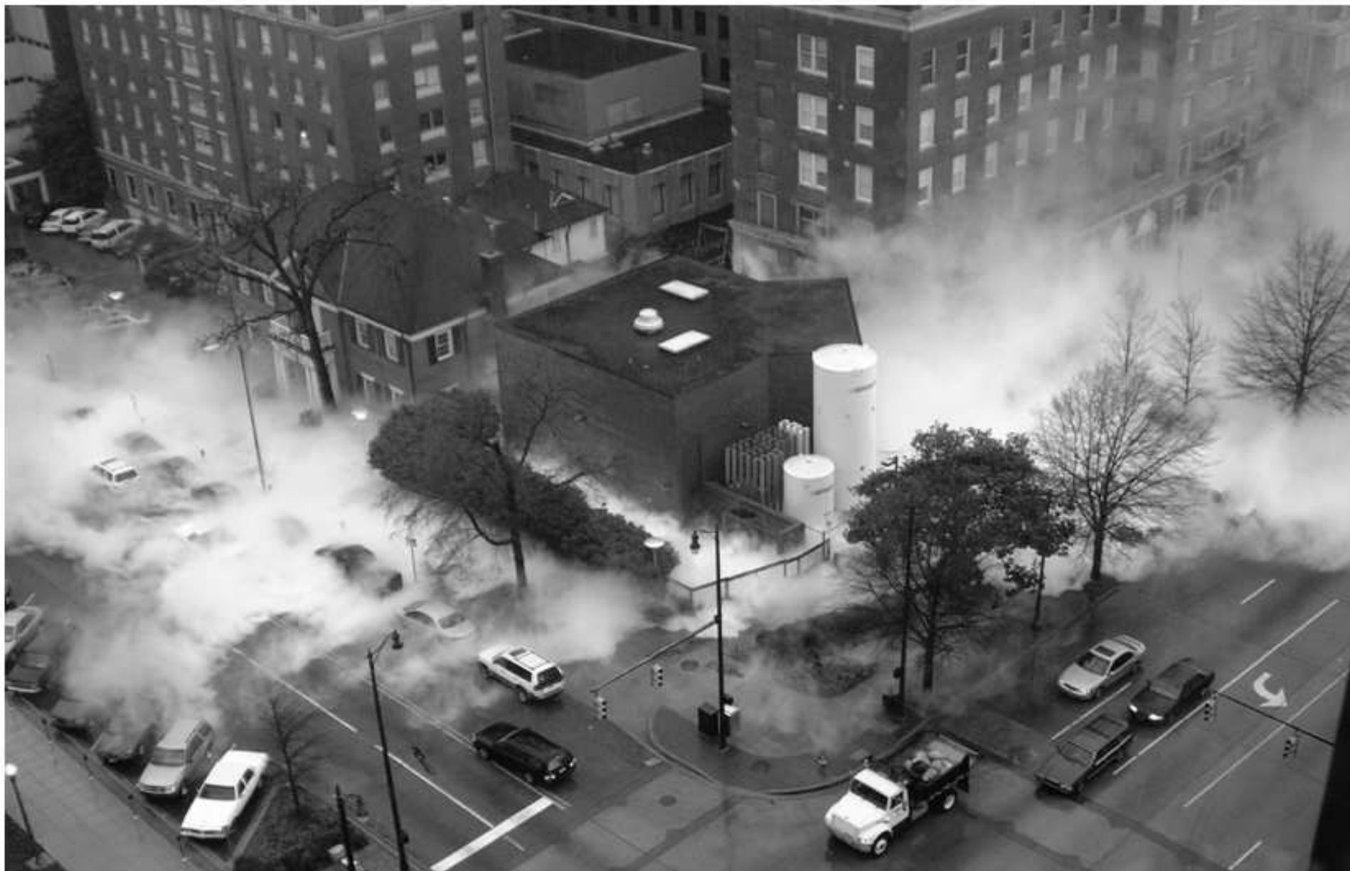
Fig. 2. Extent of the liquid oxygen leak. The main oxygen storage tank A ( right ) and the primary reserve tank B ( left ) are shown. Eight thousand gallons of liquid oxygen escaped from tank A, making it temporarily impossible for the engineers to assess either the primary or secondary reserve tank. At the time of the leak, medical center oxygen use was at a maximum, with approximately 30 operating rooms in use. At the time of this photograph, the temperature was 56°F and the relative humidity was 100%.
